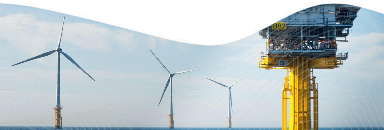
Image: Offshore High Voltage Station, Nobelwind, Belgian North Sea, Courtesy of Parkwind
